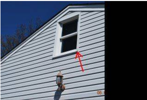
Photo 14-1 Corner of window capping loose
