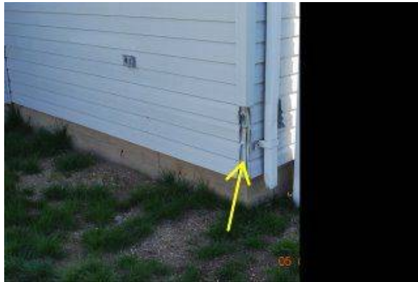
Photo 12-4 Corner siding post damaged/missing
