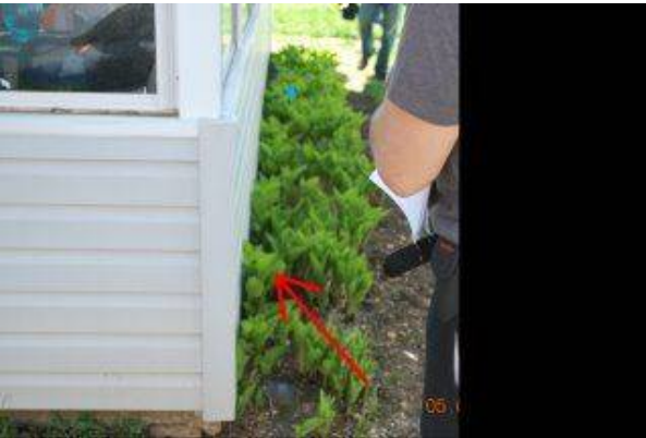
Photo 17-1 vegetation too close to building structure
