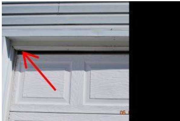
Photo 14-4 Gap at garage door very large
