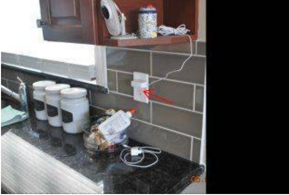
Photo 29-1 kitchen outlet not protected by GFCI and does not trip any other GFCI outlet in the area
