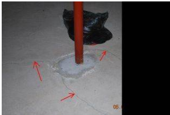
Photo 16-2 slab cracks in crawl space floor
