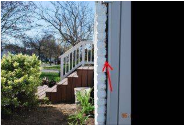
Photo 13-1 Brick Vanier pulling away from building
