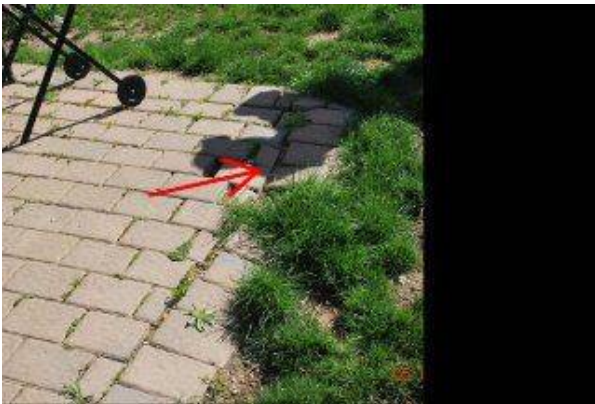
Photo 11-3 Pavers falling apart
