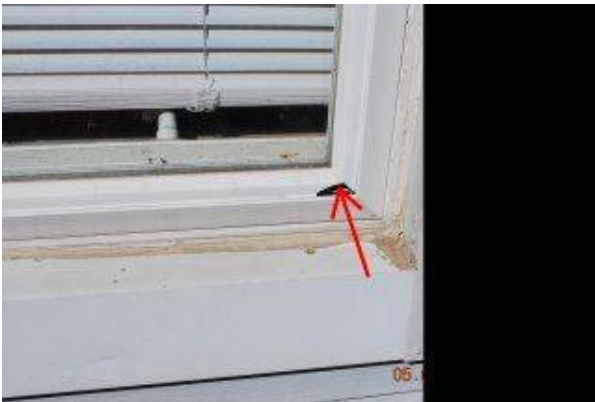
Photo 14-3 Broken window capping
