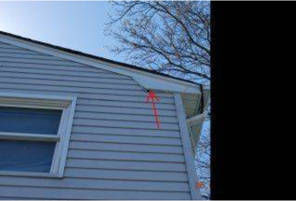
Photo 12-1 aluminum fascia cover loose
