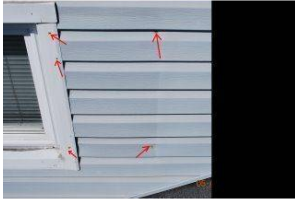
Photo 12-2 Open holes not sealed
