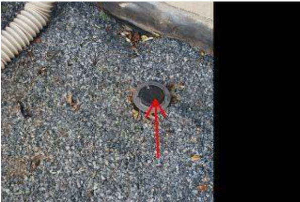
Photo 42-1 Evidence of prior Termite baiting system
