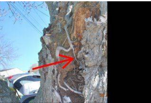
Photo 9-1 carpenter Aunt infestation at front tree
