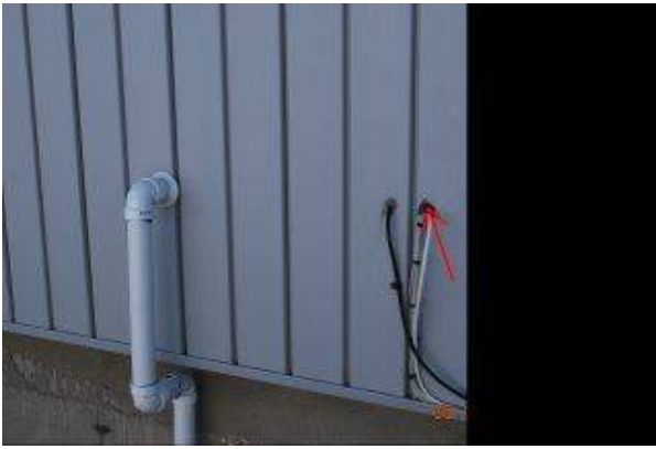
Photo 14-5 penetrations not sealed
