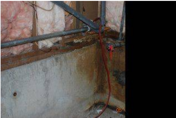
Photo 35-1 evidence of pipe corrosion
