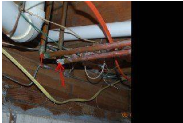
Photo 35-2 signs of corrosion at copper elbows
