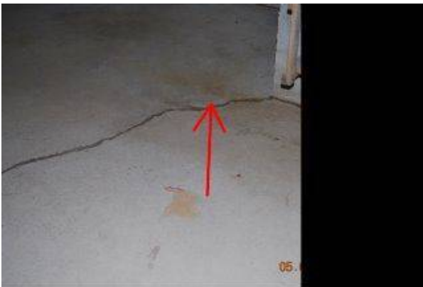
Photo 16-1 slab crack in crawl space floor
