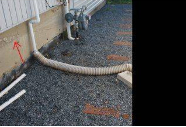
Photo 16-5 horizontal foundation cracks
