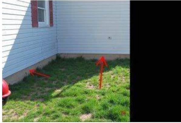
Photo 16-4 Horizontal foundation cracks
