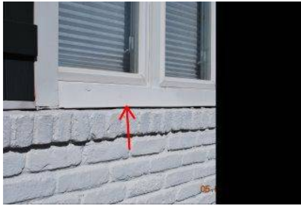
Photo 14-6 window missing caulk
