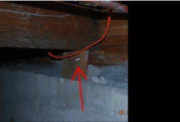
Photo 23-1 support of beam inadequate
