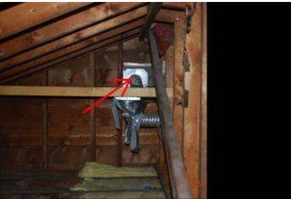
Photo 27-1 exhaust fan mounted on inside of gable vent blocking it from properly venting the attic
