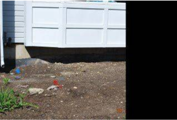
Photo 8-1 low area depression water not draining correctly
