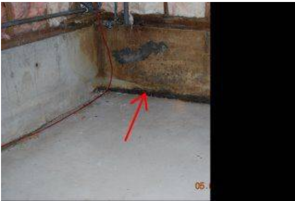
Photo 1-1 appears to be mold
