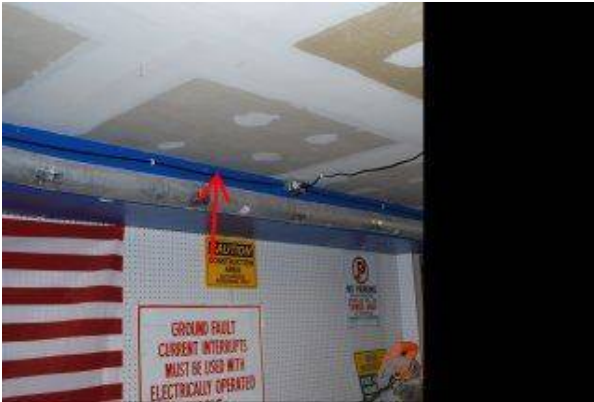
Photo 30-1 use of electrical extension cord as permeate wiring
