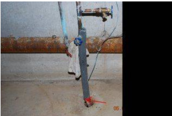
Photo 34-1 corroded grounding clamp
