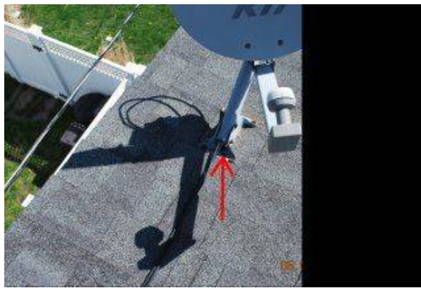
Photo 15-2 Satellite screw penetrations not caulked
