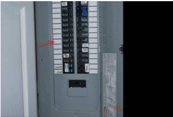
Photo 33-1 breakers missing labels
