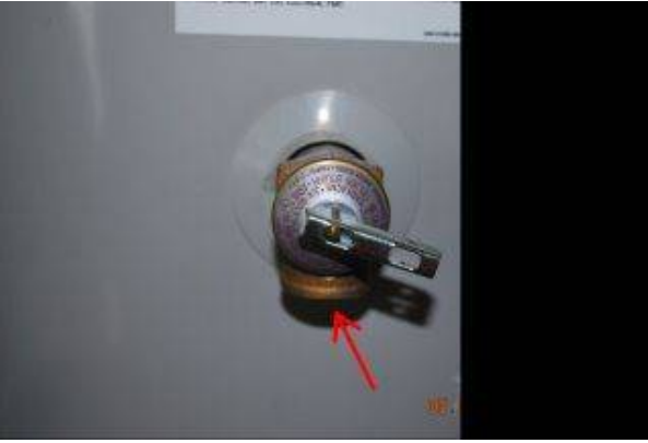
Photo 38-1 TPR valve missing discharge copper pipe
