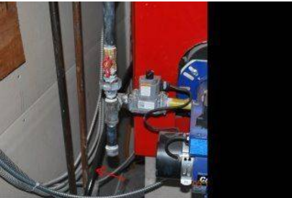
Photo 39-1 boiler drain hose made out of rubber
