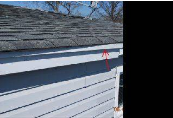
Photo 12-3 loose fascia capping
