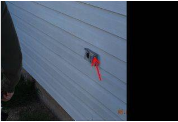
Photo 32-1 Broken exterior outlet cover
