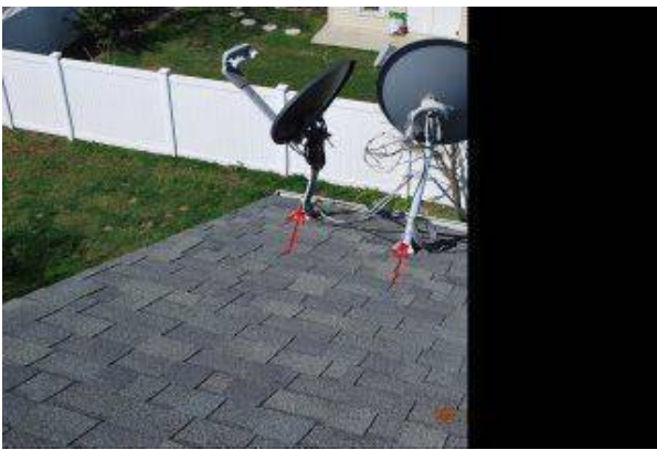
Photo 15-1 Satellite screw penetrations not caulked
