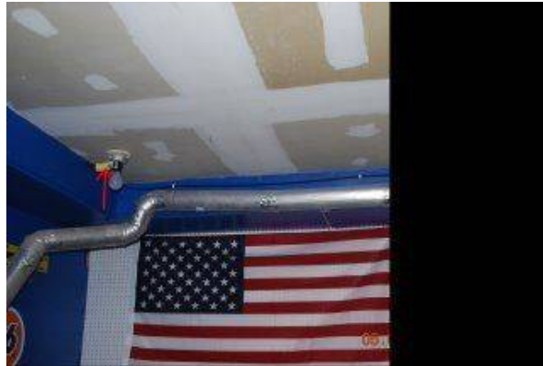
Photo 30-2 use of electrical extension cord as permeate wiring
