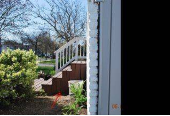
Photo 7-1 wood touching soil
