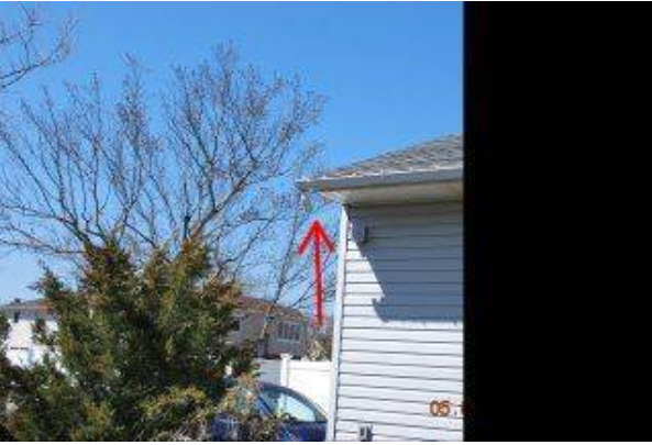
Photo 26-1 Missing section of down spout
