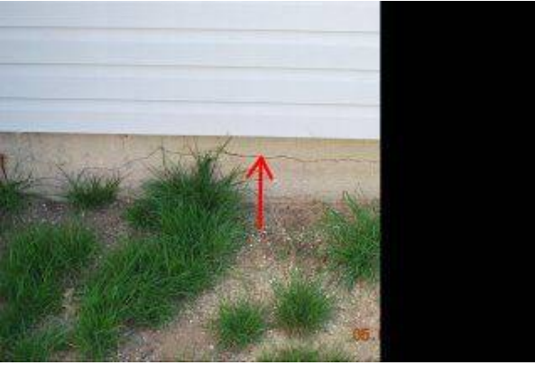
Photo 16-3 horizontal foundation cracks
